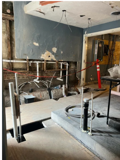
Drains and supply lines never looked so good!
