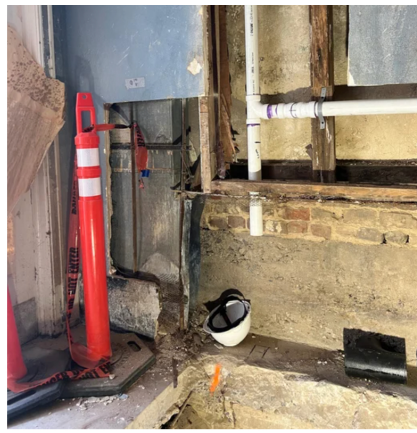
Area where covers were found - in front of the visible brickwork, behind layers of drywall (right).
